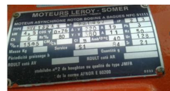
Fig.7. Wound rotor asynchronous machine nameplate
