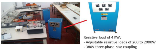
Fig.11. The performed manipulation scheme for self excitation of the induction machine (resistive load test)
